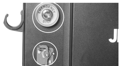
Figure.7 - Emergency Stop & Battery Isolator
