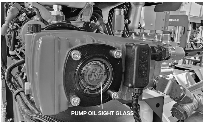
Figure.10 - Checking Pump and Gearbox Oil Level
