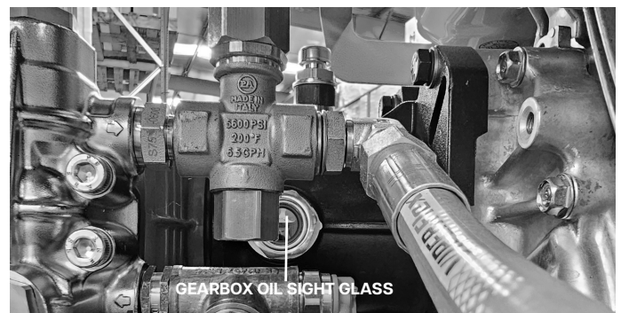
Figure.11 - Checking Pump and Gearbox Oil Level
