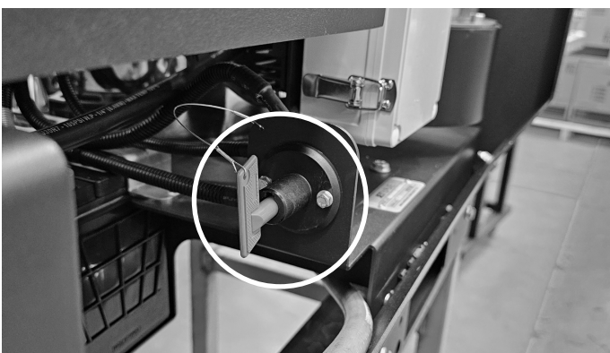
Figure.7 - Explorer G2 Battery Isolator
